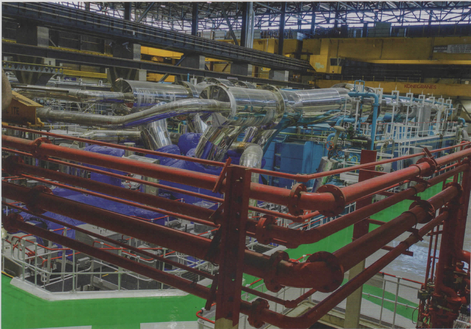
ABOVE: The Turbine Hall of Heysham 1 Power Station. BELOW: The Heysham 2 Control Room when the world record was achieved. RIGHT: John Munro the Heysham 2 Station Director.
